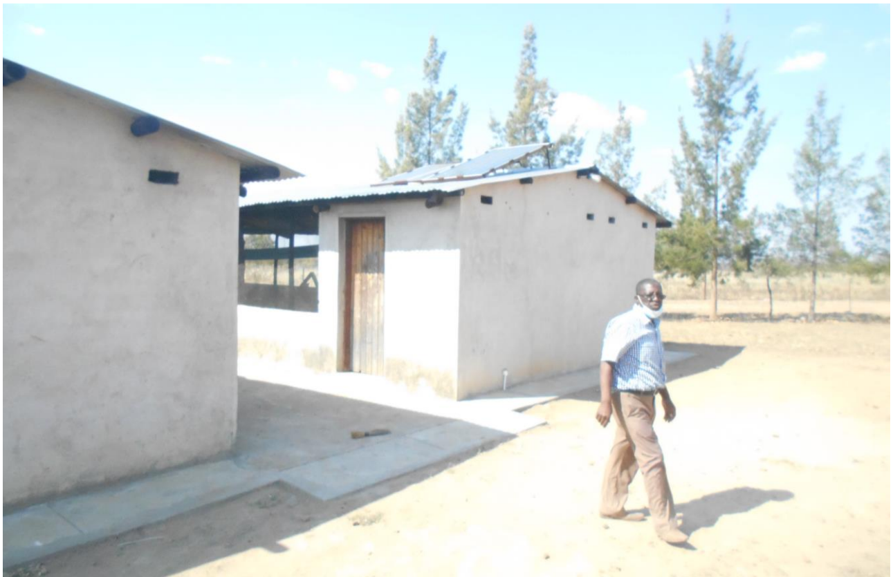
SOLAR PANELS FOR POWERING THE CENTRE ON THE FOWL-RUN'S ROOF
