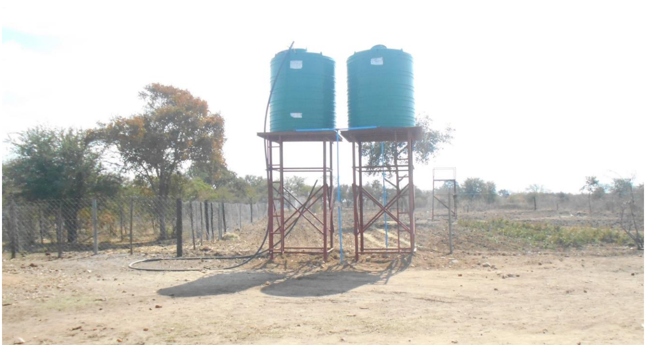
THE 2x5000 LITRES WATER TANKS FOR TRANSFIGURATION CHIDZIKWE YOUTH SKILLS TRAINING CENTRE
